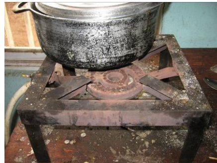
An effective functional Biogas kitchen in the SHUMAS BIOFARM Centre- Kumbo.
