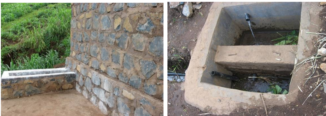
A typical water point at Tobin kumbo. And a collection chamber.
